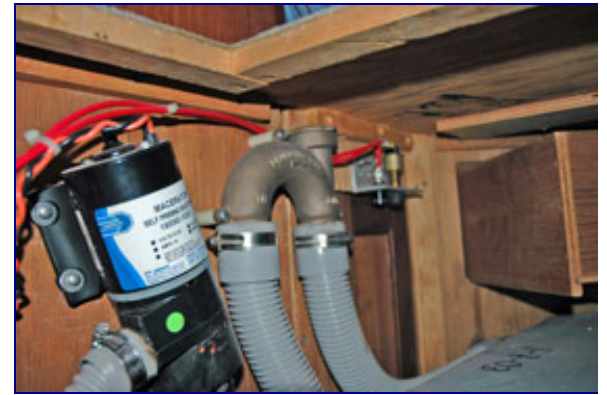
Head plumbing system
