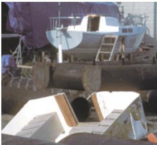
The cockpit gets cut out, above. Dave rides it to the dump, below left. The hull is gutted, below right, and gets sanded back to clean glass.
